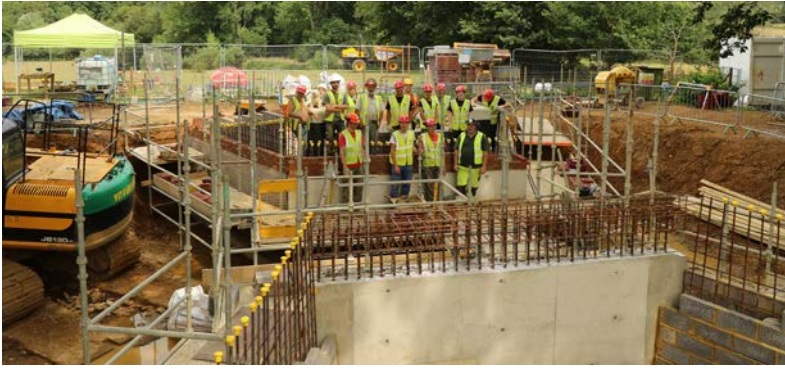
July 2019 At the end of three hot weeks of volunteer work camps, the substructure of Bridge 1 is largely complete. The brick facing was added later in the year.
