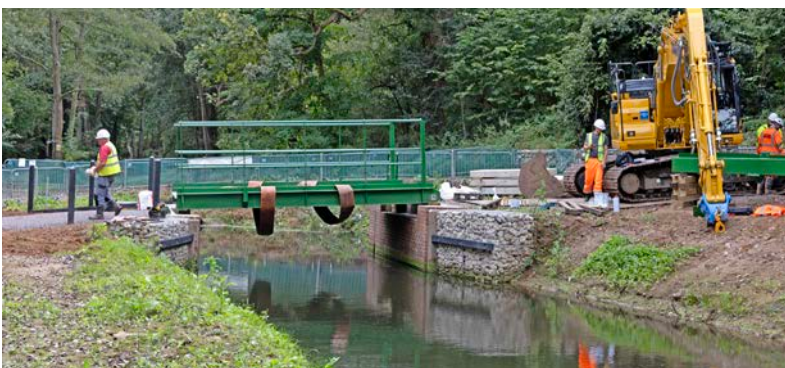
September 2023 After a challenging construction period, the substructure of Bridge 2 is complete and the lifting deck is being installed.
